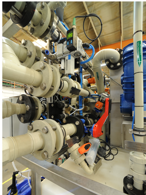
left: Detailed view MarinePaq module right: Control cabinet with touch-screen panel
