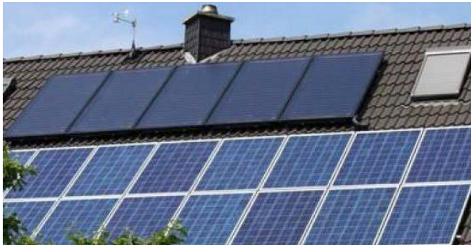
Thermal + photovoltaic panels
