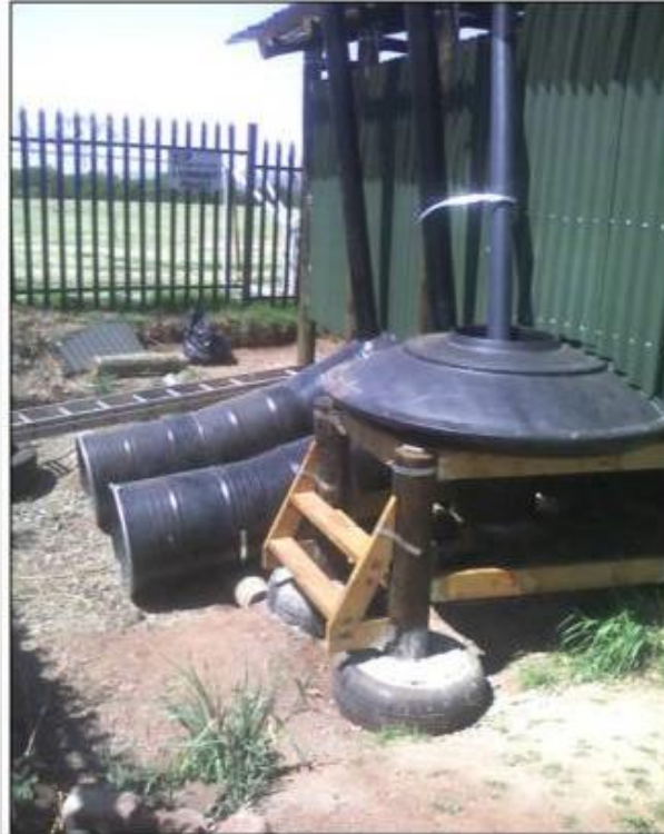
ZerH20 installation at Siyakhana Gardens, Jhb.
