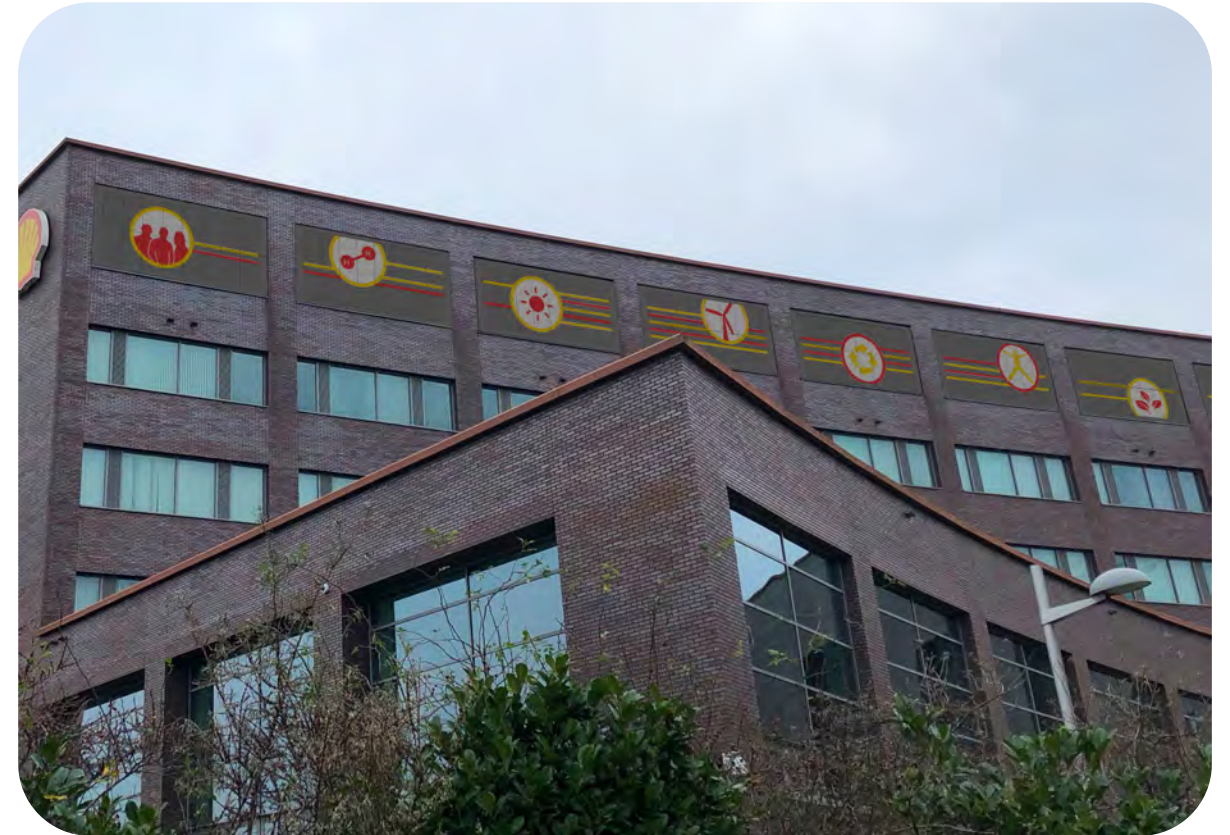
Impression Solar Visuals panels divided into 10 compartments. Each compartment is divided into 2 rows of 8 panels, size 680 x 1335 mm. Each modules contains 32 solar cells.
