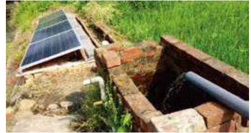
PV Water Pumping System
