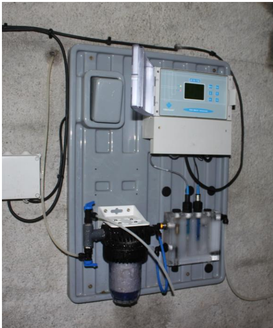
Chloride Dosing Systems
